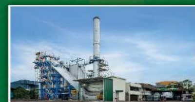
Vertical Stoker, an incinerator in Singapore, is first of its kind in South East Asia.
